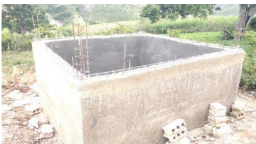
The cistern needs a new cover.
